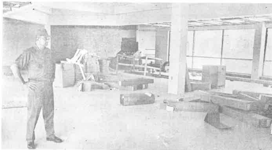
SMSgt Lou Pearman, 192d Food Services Supervisor, checks progress in the dining hall section of the new $2 million dining hall/clinic facility. The 16,080 square foot building is scheduled for completion in early September. (Photo by SSgt Dean A. Covey.)
