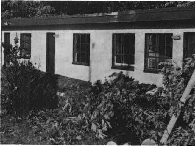
POL building sustains minor roof damage - big scare for occupants.
